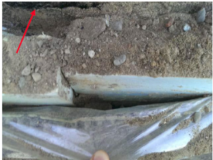
Detail view of building wall waterproofing system. Waterproofing material applied to wall (arrow) followed by rigid insulation and drainage composite layer.
