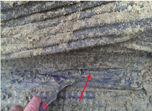
Drainage composite was not properly lapped at building wall-to-corridor roof transition. Membrane was not supported by a cant or curved fillet at the transition.
