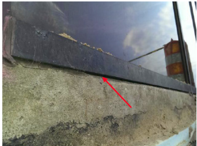
Cool interior air was flowing out of the building along storefront glazing sill at the 1st floor slab surface.
