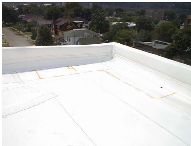
Overview of wet insulation identified during the StructureScan® survey.
